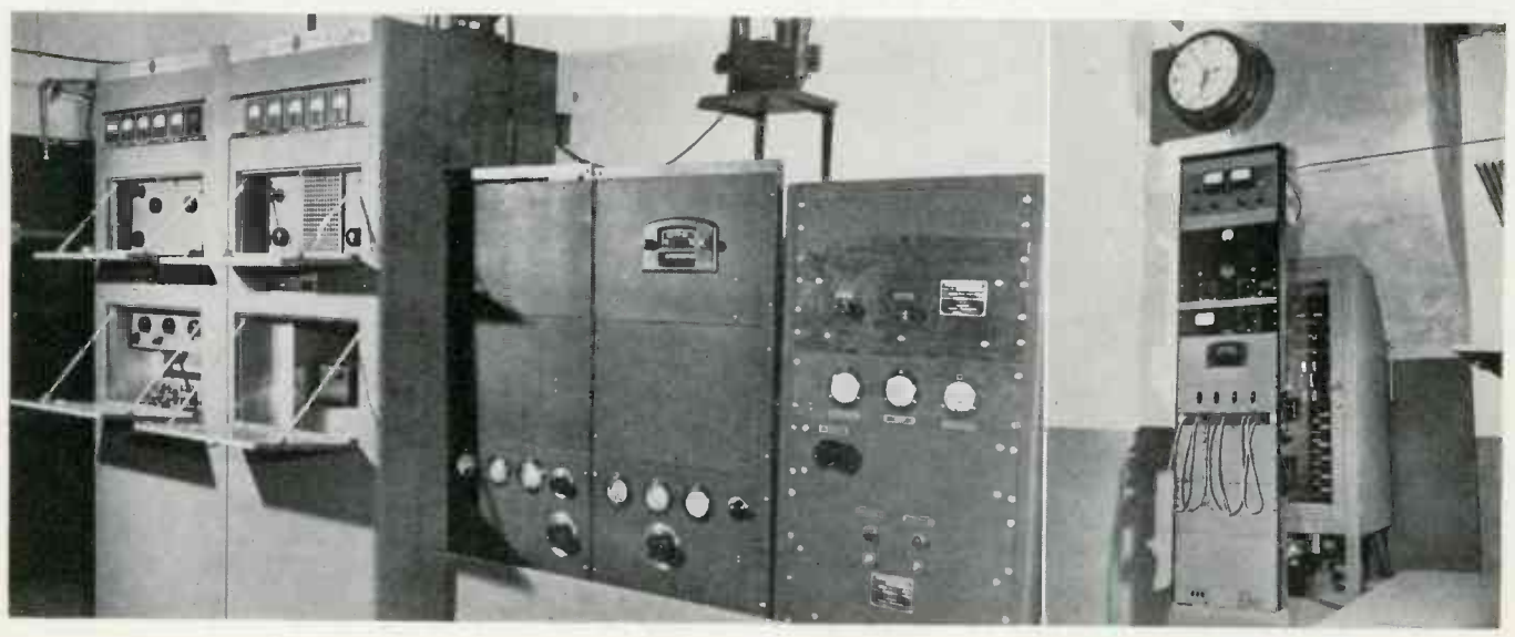
The new FM transmitter is installed alongside a television transmitter. At the right are the FM transmitter for television sound, and the video modulator. Separate picture at extreme right shows speech input for FM transmitter
